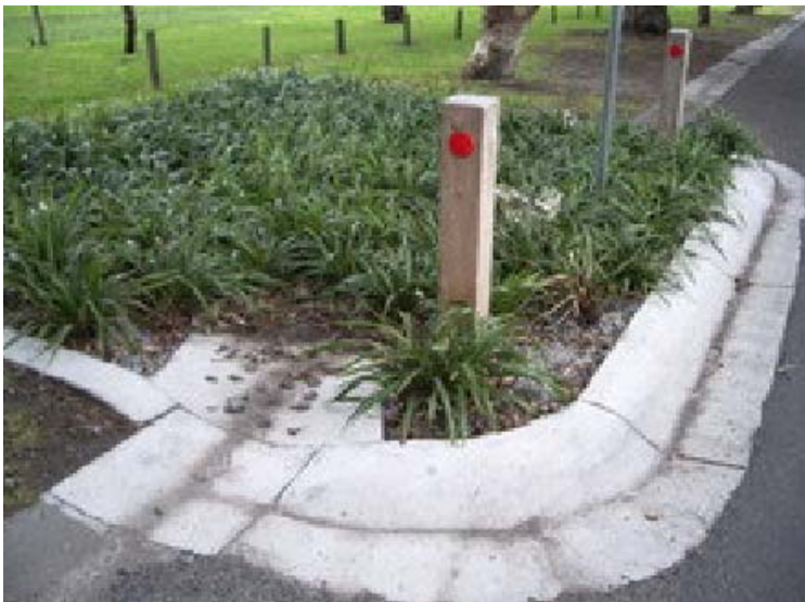
FIGURE 5-8 : KERB INLETS TO SMALL SCALE BIORETENTION SYSTEM (SOURCE: CITY OF KINGSTON)
